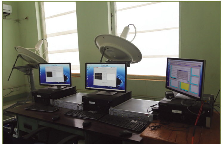
Figure 8.3: Dual frequency beacon receiver installed at NESAC
