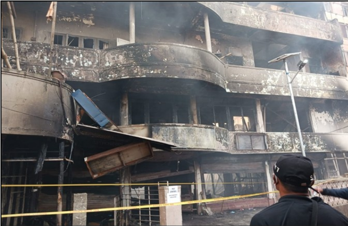
Fire Incident- Janata Furniture Building from ground zero on 15.10.2023
